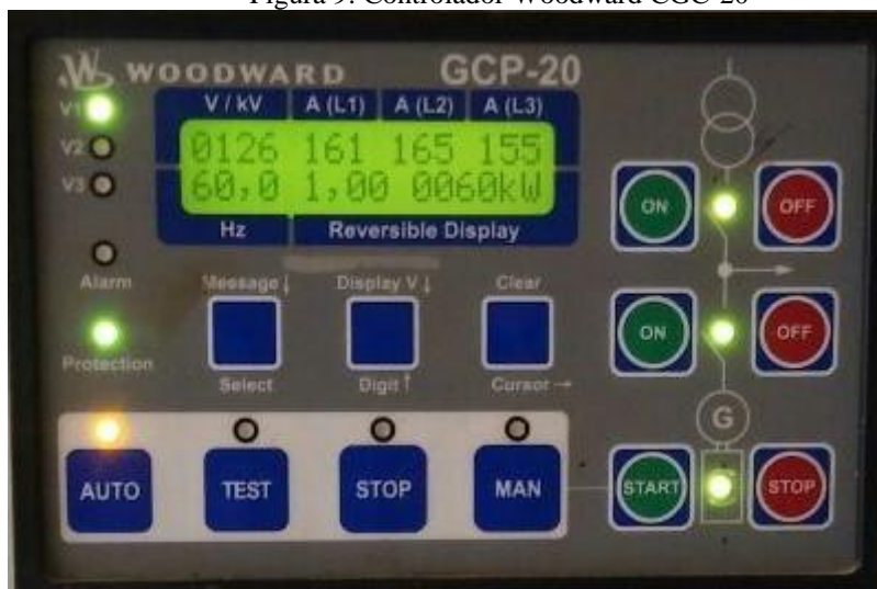
Figura 9: Controlador Woodward CGC-20
